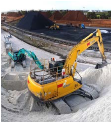
Gypsum is imported through Fremantle Ports' Kwinana Bulk Terminal. It is used for making plasterboard.
