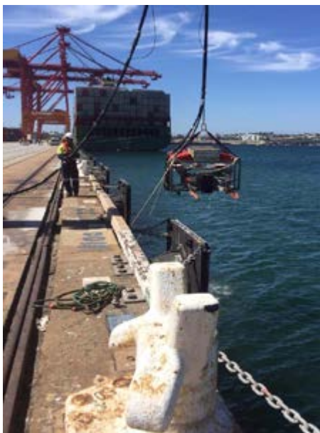
A Diamond Wire Saw, a hydraulically powered, remotely operated pile cutter, is used to cut piles at the seafloor, removing the need to have divers in the water to manually cut the piles.
