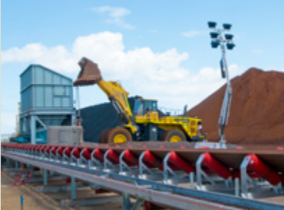
New export conveyor at the Kwinana Bulk Terminal
