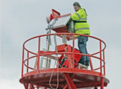
Navigational lighting maintenance is an essential element of asset management.
